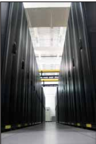
Our DFT facility located in Elk Grove, IL is one of the Midwest's most sophisticated and efficient data centers.
