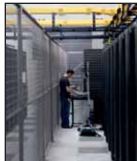
On-site, industry certified technical staff monitor and inspect data center facilities 24/7.
